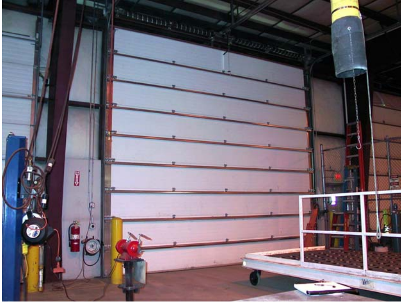
Photo 1. The overhead door that was involved in the fatal incident: a standard lift steel insulated door with six-inch lift drums. The door in the photo was adjusted and repaired by a garage door technician after the incident.
