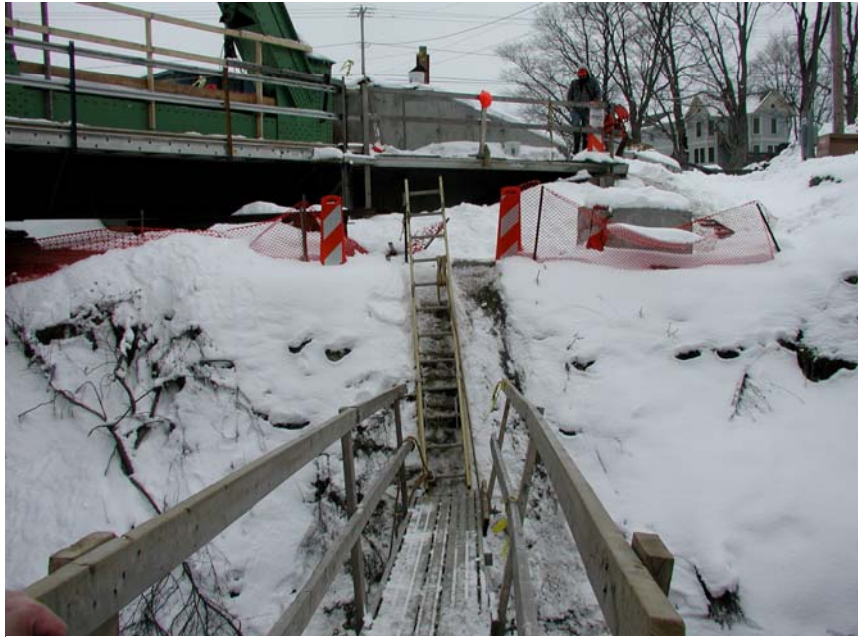
Photo 3. The ladder and catwalk that served as the only entrance to the barge.
