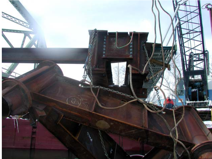
Photo 5. The pile cap hung by the test chains after it broke apart from the W36 I-beams.
