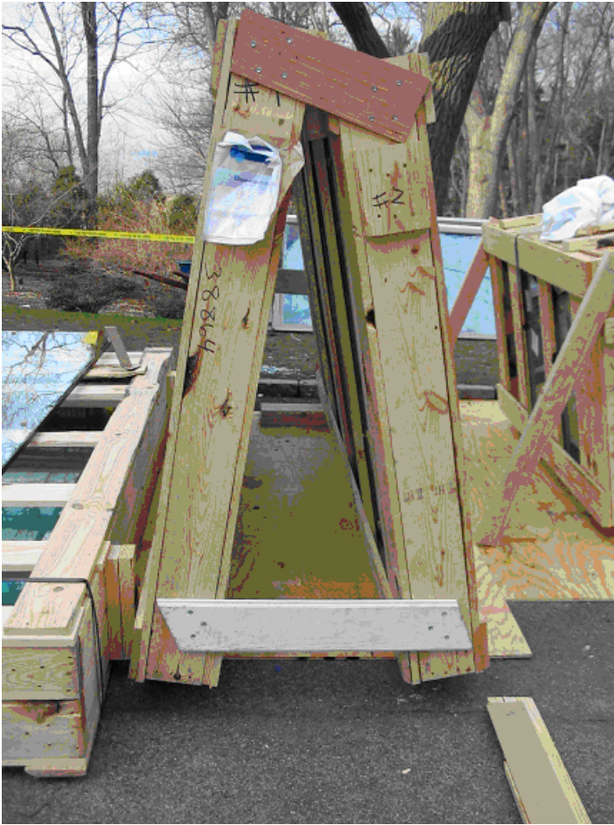
Photo 1 (courtesy of OSHA). The first “A” frame that was set up by the workers. The smaller crate supported by the two wooden bars is on the right.
