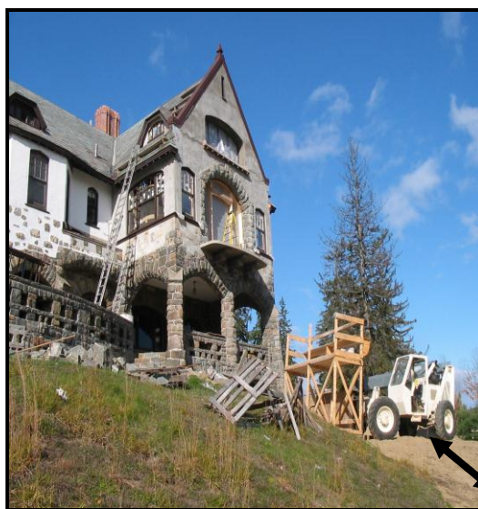
Photo 2 Sloped terrain (courtesy of OSHA)
